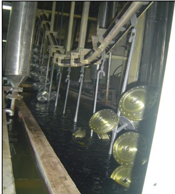
Pic: Top surface not insulated
